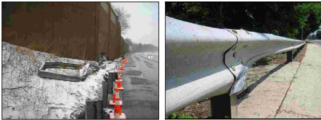
Fig. 1. Does the damage to these w-beam barriers hinder their performance
