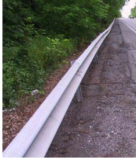
Figure 3 – Weak Post W-Beam Barrier (NASS/CDS Case 2002-002-041)
