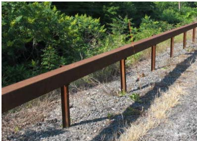
Figure 5 – Box-Beam Barrier (NASS/CDS Case 2007-002-071)
